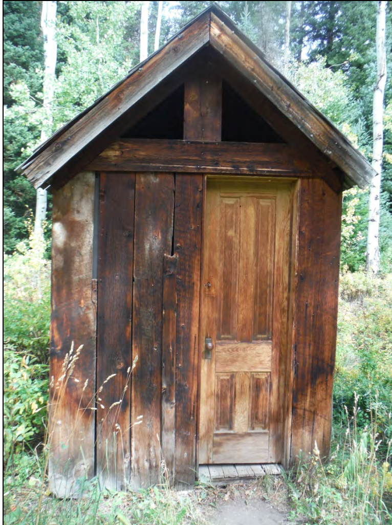
5GN6536 – Clayton Cabin. View of the south elevation of the outhouse. View north. (Roll 19-259, image 516, 09/26/2019)
