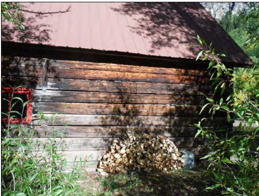
5GN6529 – Rosetta Cabin. View of east elevation including north end. View west. (Roll 19-260, image 614, 09/27/2019)
