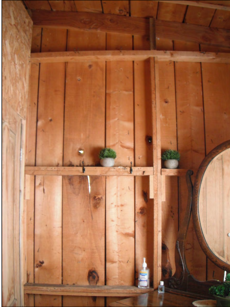
5GN6529 – Rosetta Cabin. View of the interior of the bathhouse. View east. (Roll 19-261, image 194, 09/27/2019)
