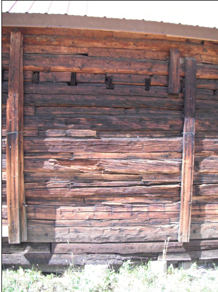
5GN6527 – Crystal Club. Detail of east elevation showing the ends of the interior floor joists exposed on the exterior. View west. (Roll 19-261, image 147, 09/27/2019)
