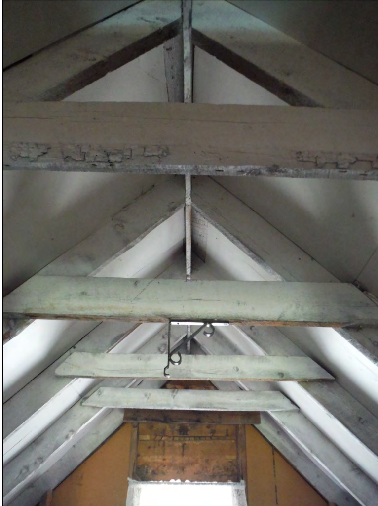
5GN6529 – Rosetta Cabin. Interior of the cabin, detail of framing inside the roof peak. View north. (Roll 19-260, image 697, 09/27/2019)
