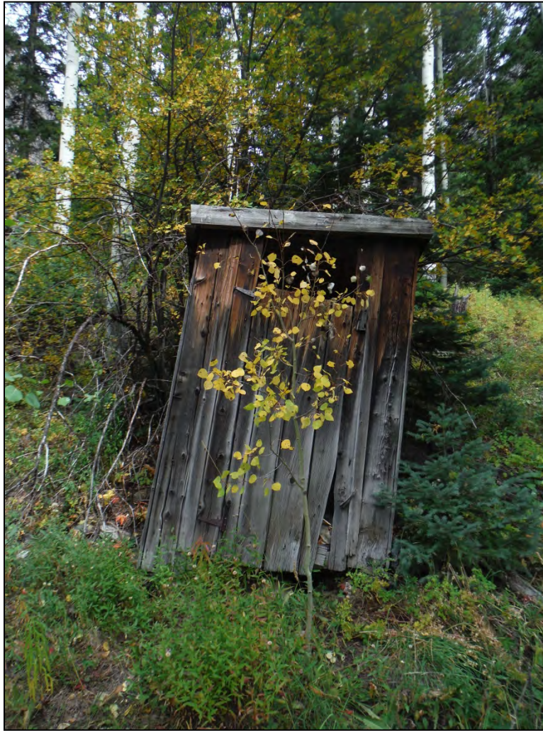
5GN6535 – Melton House. View of the south elevation of the outhouse. View north. (Roll 19-259, image 531, 09/26/2019)
