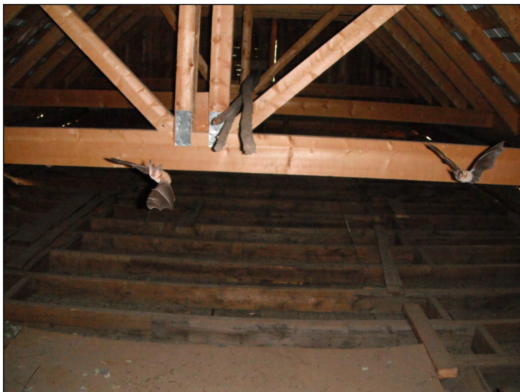
5GN6527 – Crystal Club. Interior, view of the new roof trusses above the main room of the original building, also showing original floor joists and current residents. View north. (Roll 19-262, image 286, 09/27/2019)
