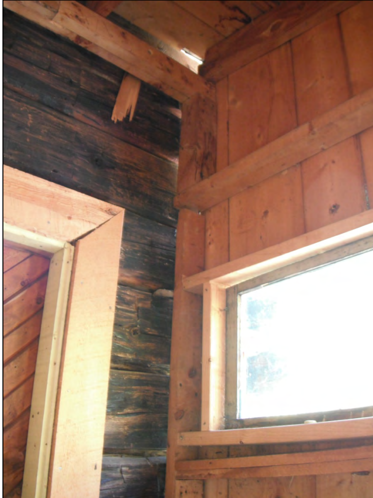
5GN6529 – Rosetta Cabin. Detail of the interior juncture of the main cabin with the added bathhouse. View northeast. (Roll 19-261, image 192, 09/27/2019)
