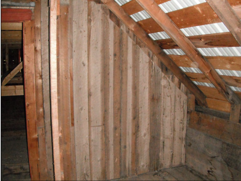
5GN6527 – Crystal Club. Interior, view of the northeast corner of the east second floor room above the addition, also showing the new roof framing. View northeast. (Roll 19-262, image 293, 09/27/2019)
