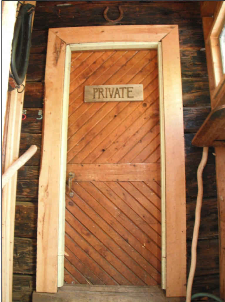
5GN6529 – Rosetta Cabin. View of the back door that leads into the cabin from inside the bathhouse door. View north. (Roll 19-261, image 198, 09/27/2019)
