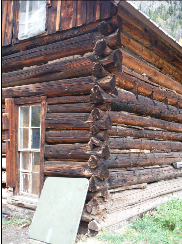
5GN6528 – General Store. Detail of steep log notching on southeast corner. View northwest. (Roll 19-260, image 730, 09/27/2019)
