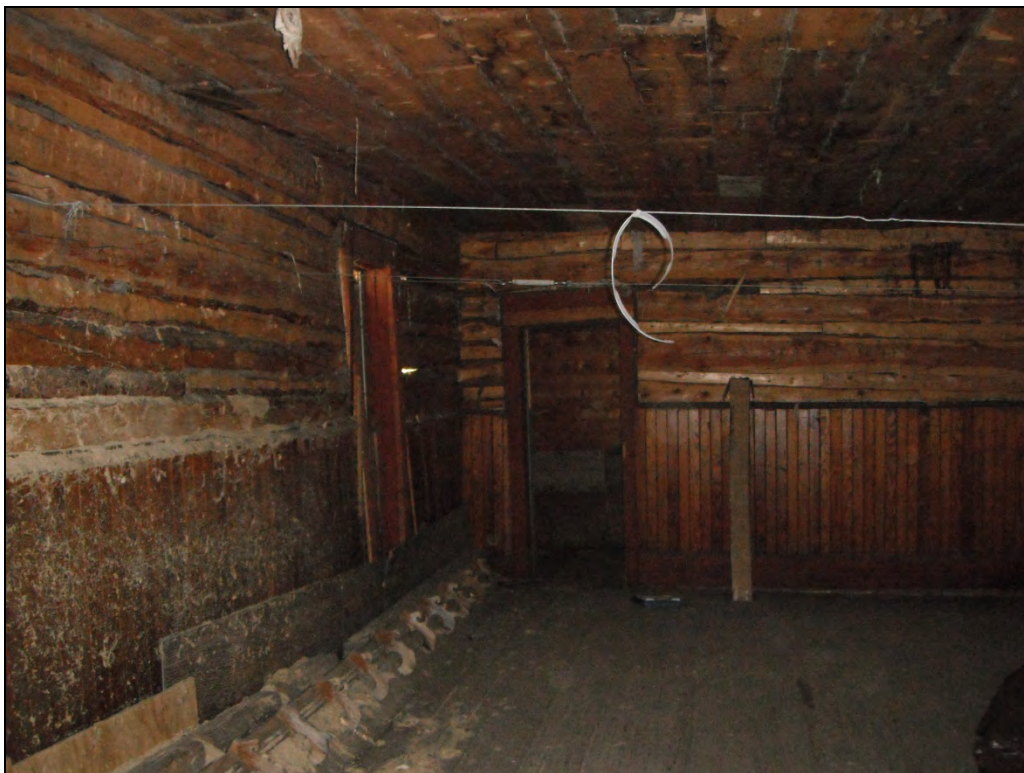
5GN6527 – Crystal Club. Interior, view of the southeast corner of the main ground floor room in the original building. View southeast. (Roll 19-262, image 278, 09/27/2019)
