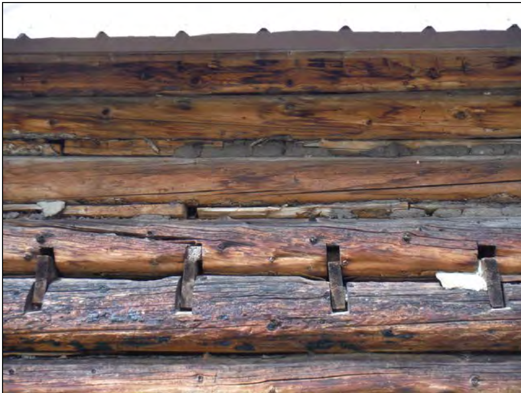
5GN6528 – General Store. Detail of interior floor joist ends visible on the east elevation. View northwest. (Roll 19-260, image 734, 09/27/2019)
