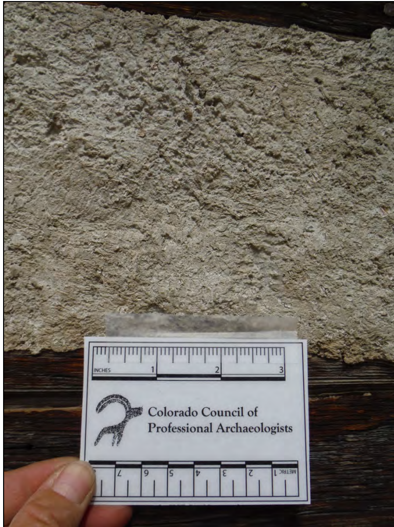
5GN6536 – Clayton Cabin. Detail of fibrous mud chinking used on the exterior of the cabin. (Roll 19-259, image 552, 09/26/2019)
