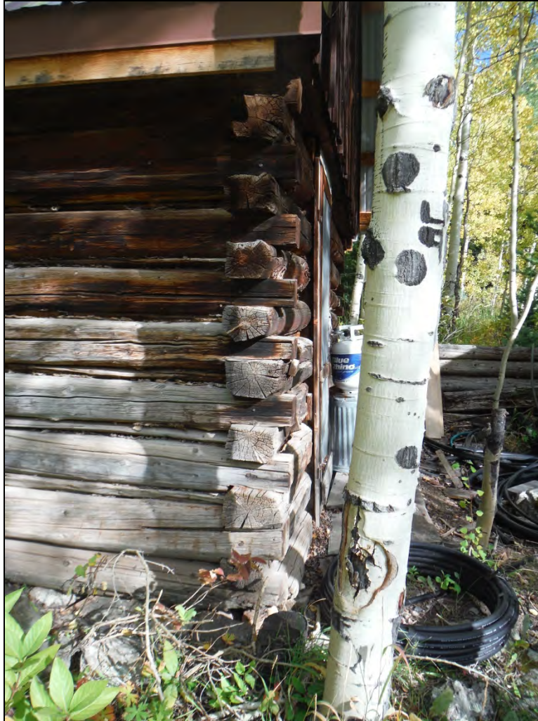
5GN6530 – Edgerton Cabin. Detail of log notching on southwest corner. View northeast. (Roll 19-259, image 594, 09/26/2019)
