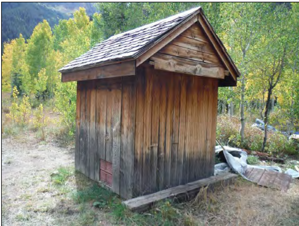
5GN6528 – General Store. Oblique view of the northwest corner of the outhouse. View southeast. (Roll 19-260, image 739, 09/27/2019)
