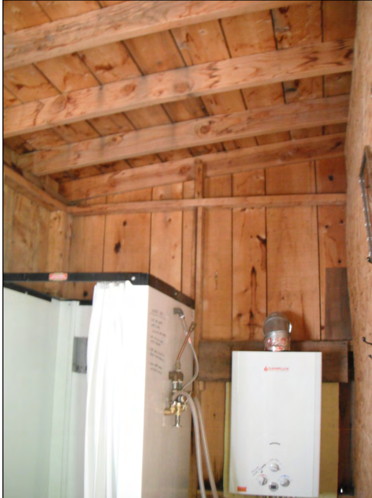
5GN6529 – Rosetta Cabin. View of the interior of the bathhouse. Note shower and water heater. View west. (Roll 19-261, image 193, 09/27/2019)
