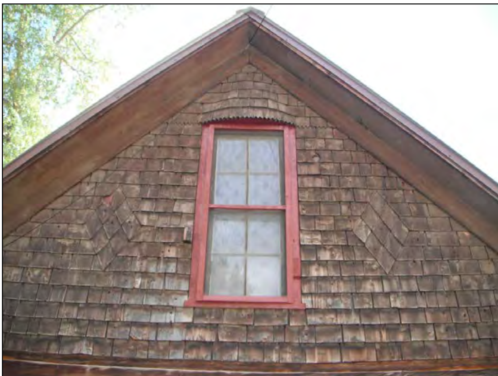
5GN6529 – Rosetta Cabin. Detail of decorative shingle pattern and eyebrow dormer in the gable on the north elevation. View south. (Roll 19-261, image 179, 09/27/2019)
