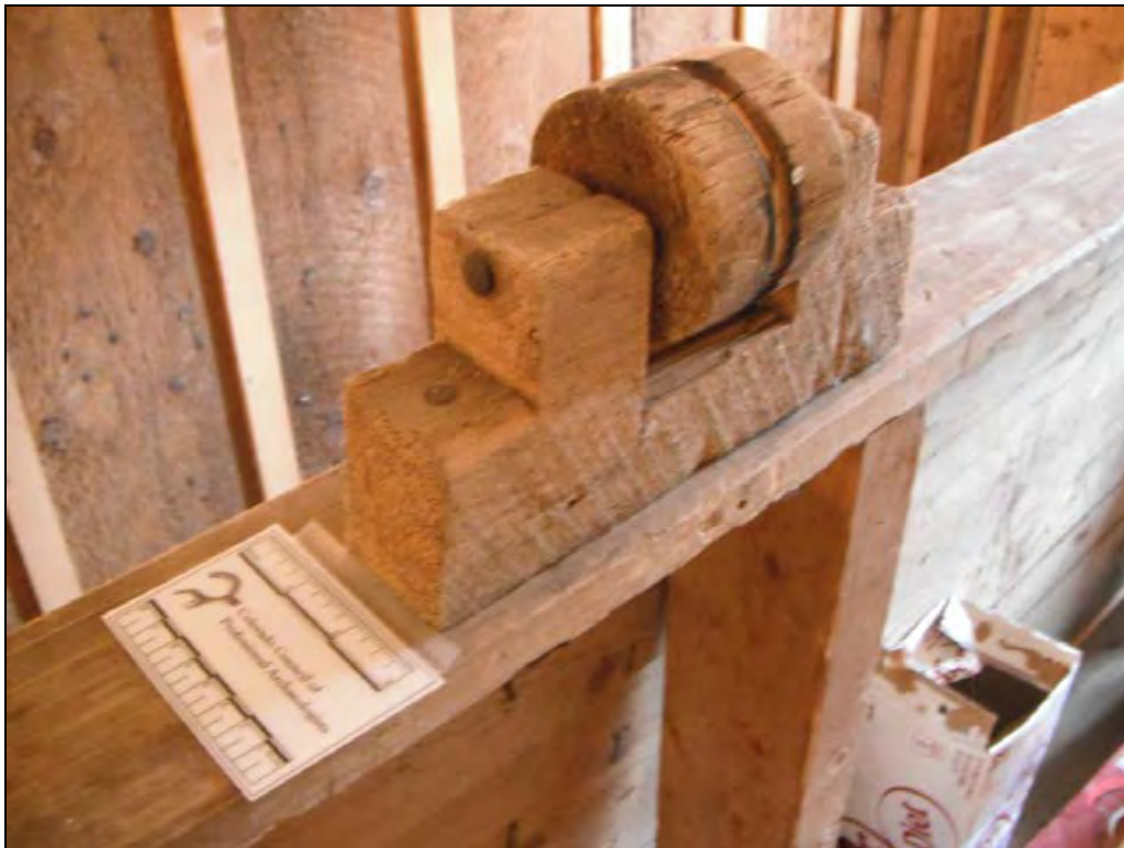
5GN6528 – General Store. View of the interior, original pulley mechanism located on the handrail at the top of the stairs. View southeast/plan. (Roll 19-261, image 239, 09/27/2019)
