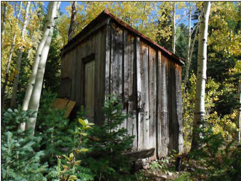
5GN6530 – Edgerton Cabin. Oblique view of the northwest corner of the shed. View southeast. (Roll 19-259, image 604, 09/26/2019)
