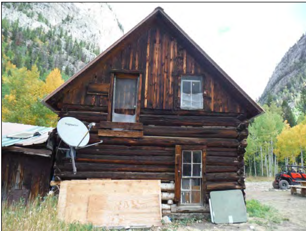
5GN6528 – General Store. Detail of south elevation of the main cabin. Note new aspen logs added to the west of the ground floor window. View north. (Roll 19-260, image 724, 09/27/2019)
