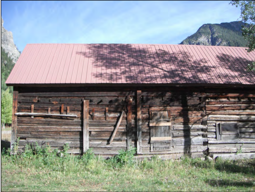
5GN6527 – Crystal Club. View of west elevation including north end. View east. (Roll 19-258, image 61, 09/25/2019)
