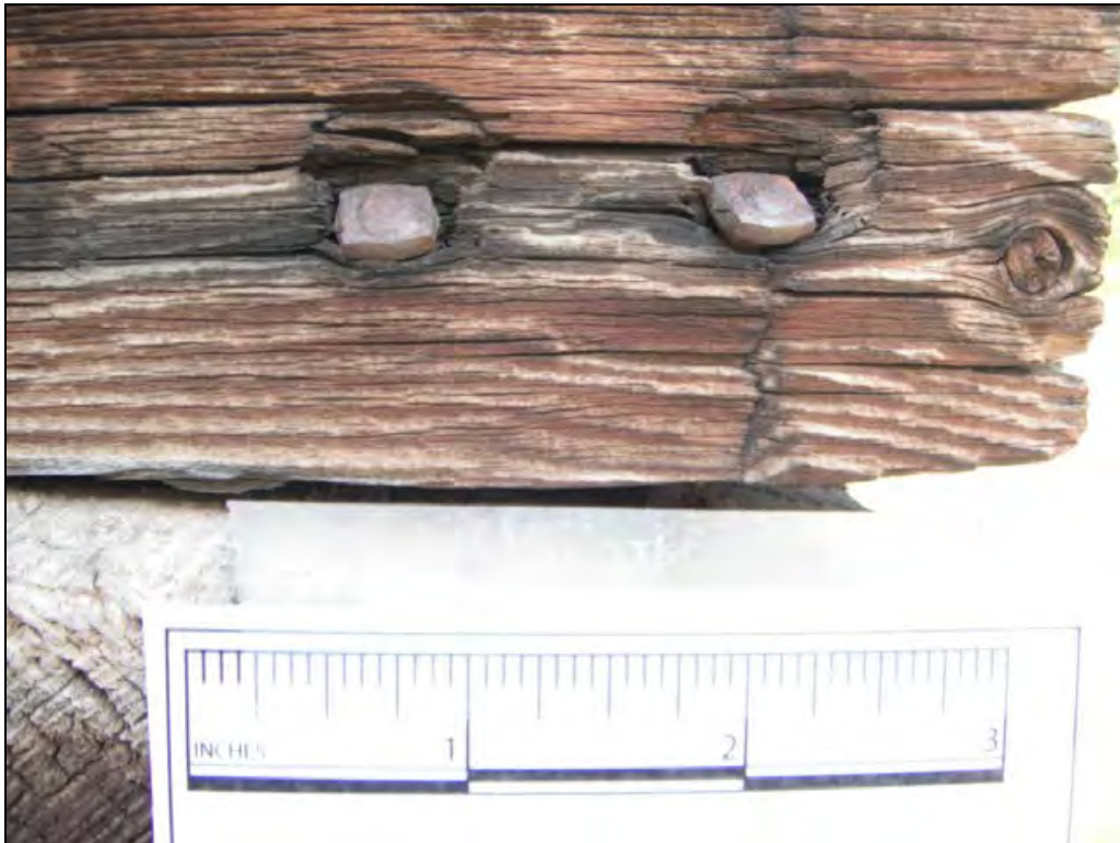
5GN6529 – Rosetta Cabin. Detail of square nails used in the construction of the cabin at the northwest corner. View south. (Roll 19-261, image 176, 09/27/2019)
