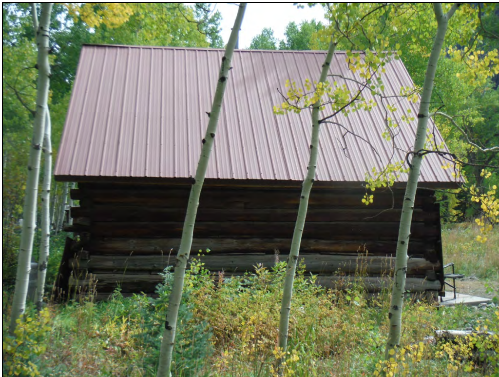
5GN6536 – Clayton Cabin. View of the west elevation. View east. (Roll 19-259, image 514, 09/26/2019)
