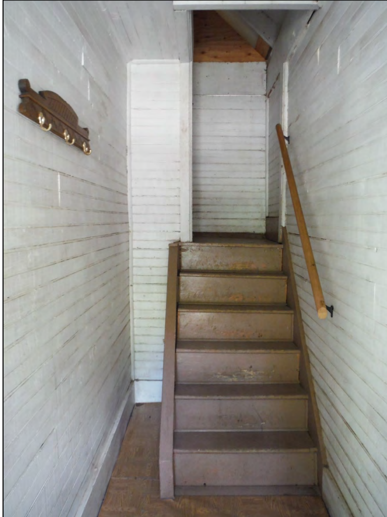
5GN6529 – Rosetta Cabin. Interior of the cabin, view of entryway and first set of stairs leading up to the second story. View south. (Roll 19-260, image 686, 09/27/2019)
