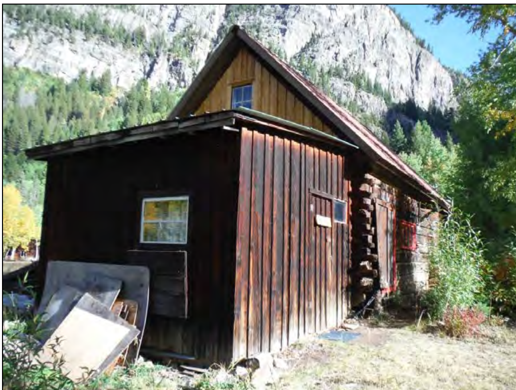
5GN6529 – Rosetta Cabin. Oblique view of southeast corner. View northwest. (Roll 19-260, image 612, 09/27/2019)
