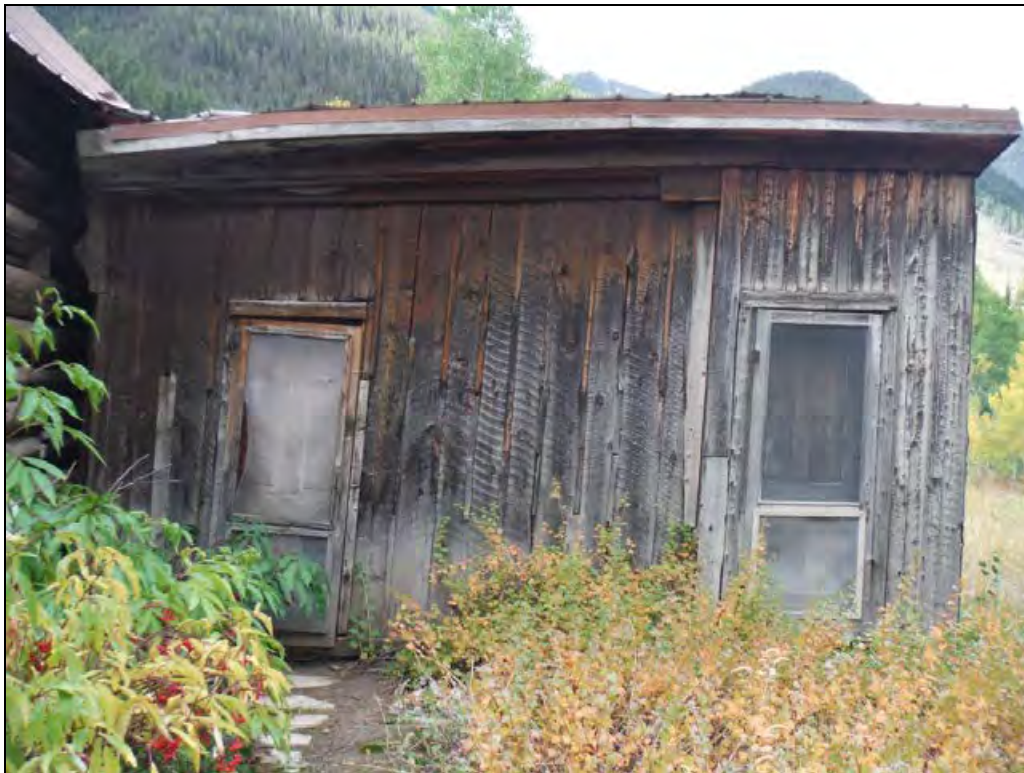
5GN6528 – General Store. Detail of the north elevation of the addition. View south. (Roll 19-260, image 707, 09/27/2019)
