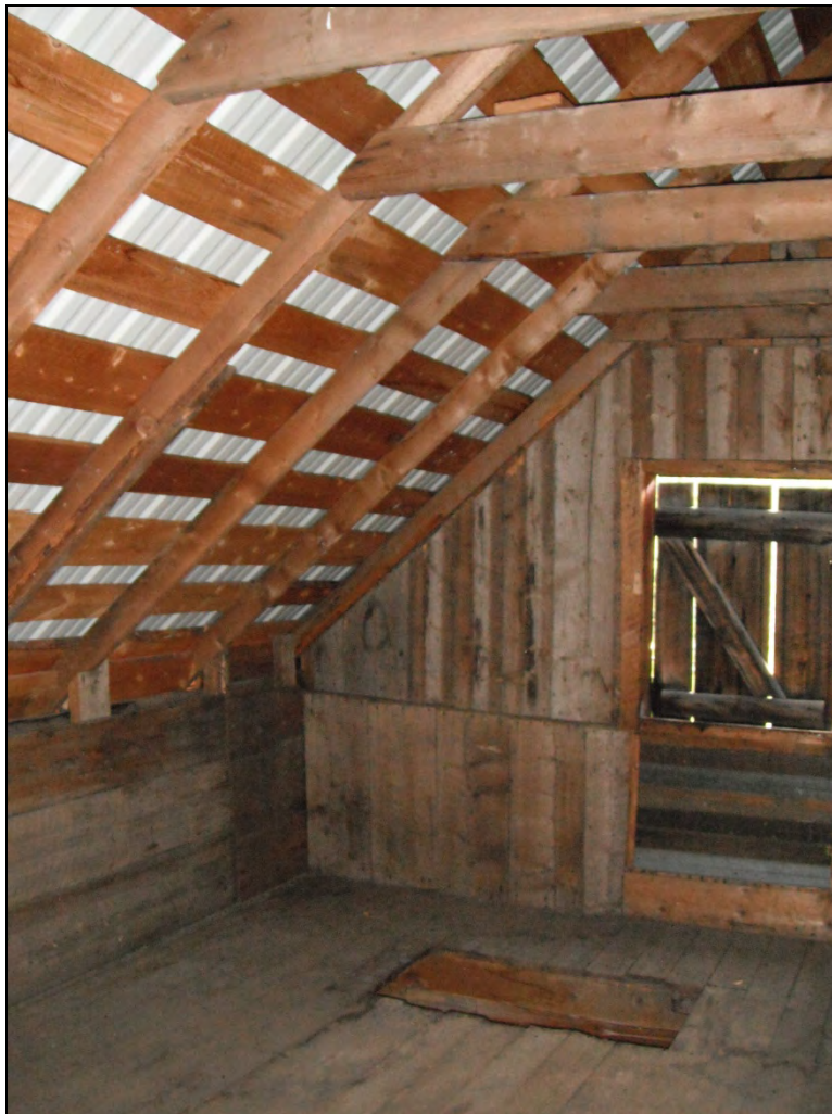
5GN6527 – Crystal Club. Interior, view of the southeast corner of the east second floor room above the addition, also showing the new roof framing. View southeast. (Roll 19-262, image 287, 09/27/2019)
