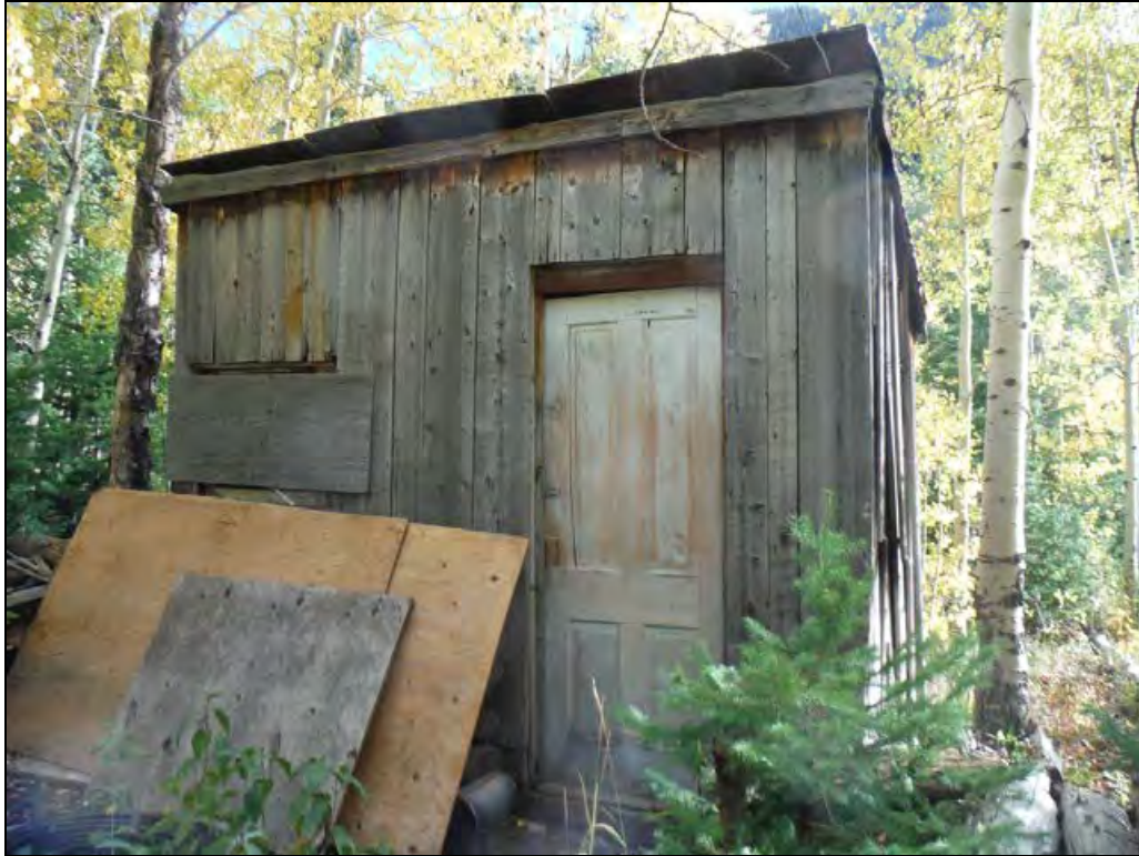
5GN6530 – Edgerton Cabin. View of the north elevation of the shed. View south. (Roll 19-259, image 603, 09/26/2019)
