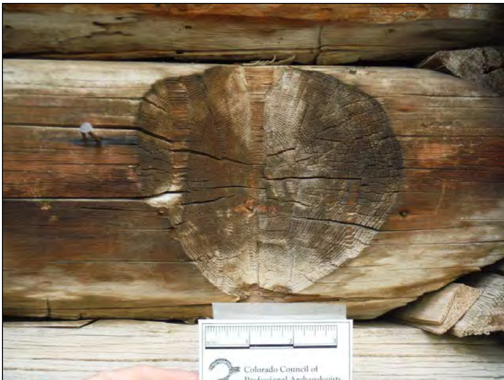
5GN6530 – Edgerton Cabin. Detail of notch in the log on the north elevation which is visible in an historic photo (Neal 2002:27). View south. (Roll 19-260, image 747, 09/27/2019)
