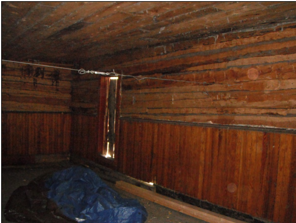
5GN6527 – Crystal Club. Interior, view of the southwest corner of the main ground floor room in the original building. View southwest. (Roll 19-262, image 277, 09/27/2019)
