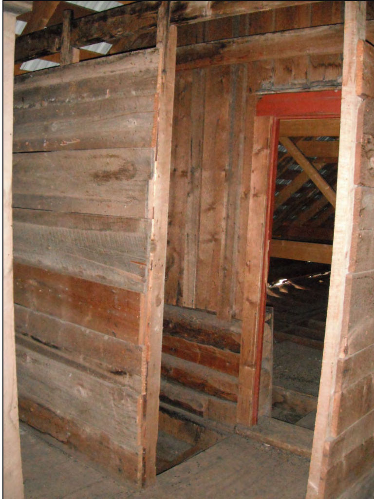
5GN6527 – Crystal Club. Interior, view of the head of the stairs in the addition from the east second floor room. View northwest. (Roll 19-262, image 290, 09/27/2019)
