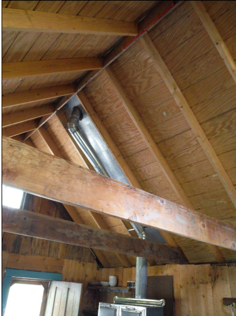
5GN6530 – Edgerton Cabin. View of the interior of the cabin showing stovepipe and new roof. View northeast/up. (Roll 19-260, image 670, 09/27/2019)
