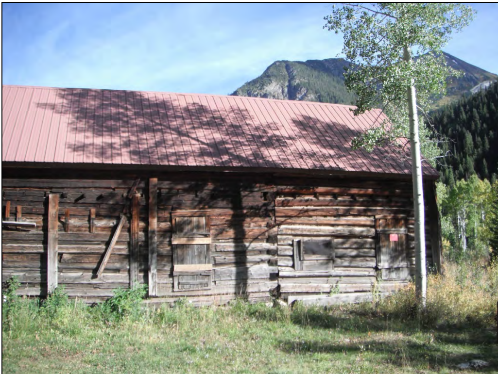
5GN6527 – Crystal Club. View of west elevation including south end. View east. (Roll 19-258, image 62, 09/25/2019)
