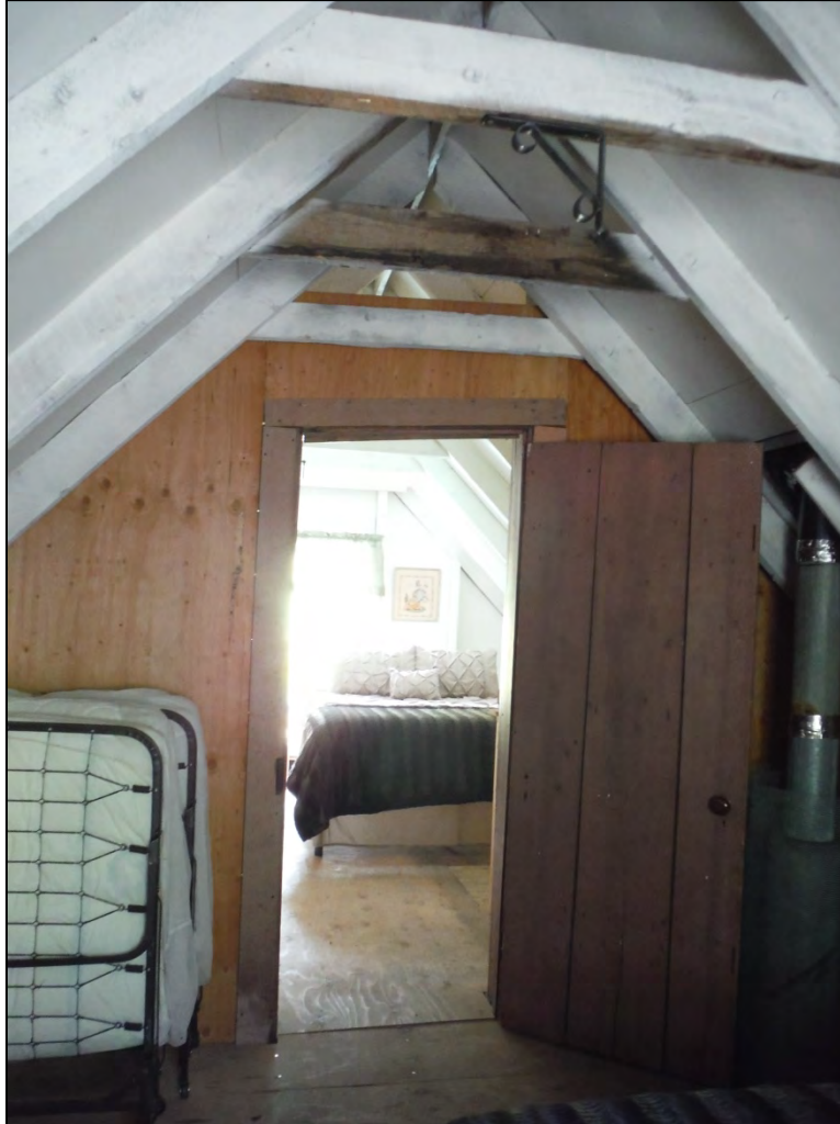
5GN6529 – Rosetta Cabin. Interior of the cabin, view from the north bedroom into the south on the second story. View south. (Roll 19-260, image 695, 09/27/2019)
