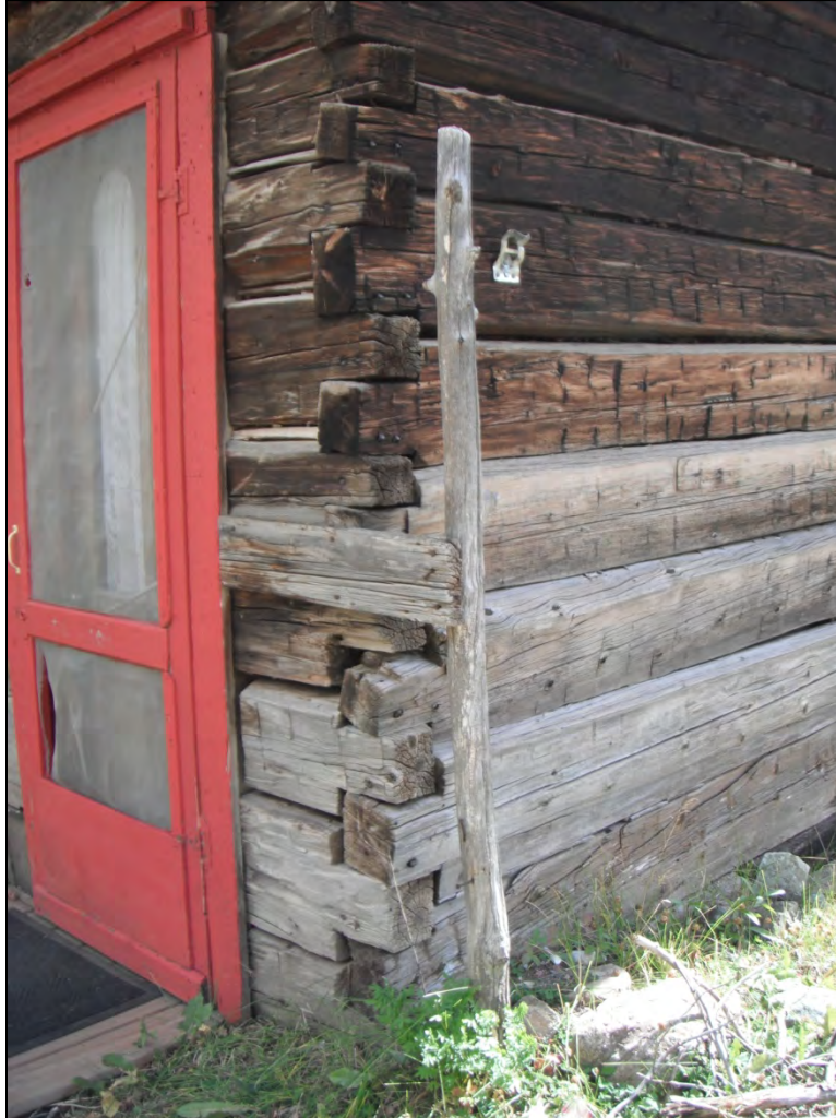
5GN6529 – Rosetta Cabin. Detail of square log notching on northwest corner. View southeast. (Roll 19-261, image 185, 09/27/2019)
