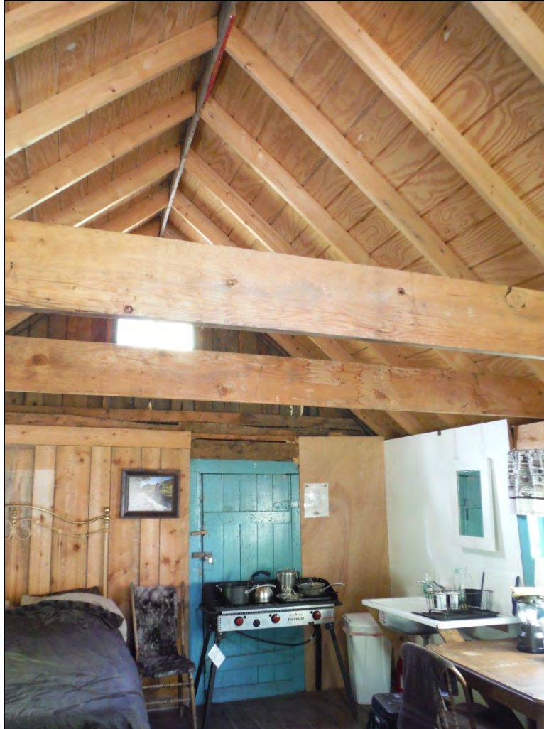
5GN6530 – Edgerton Cabin. View of the interior of the cabin showing new roof. View south-southwest/up. (Roll 19-260, image 672, 09/27/2019)
