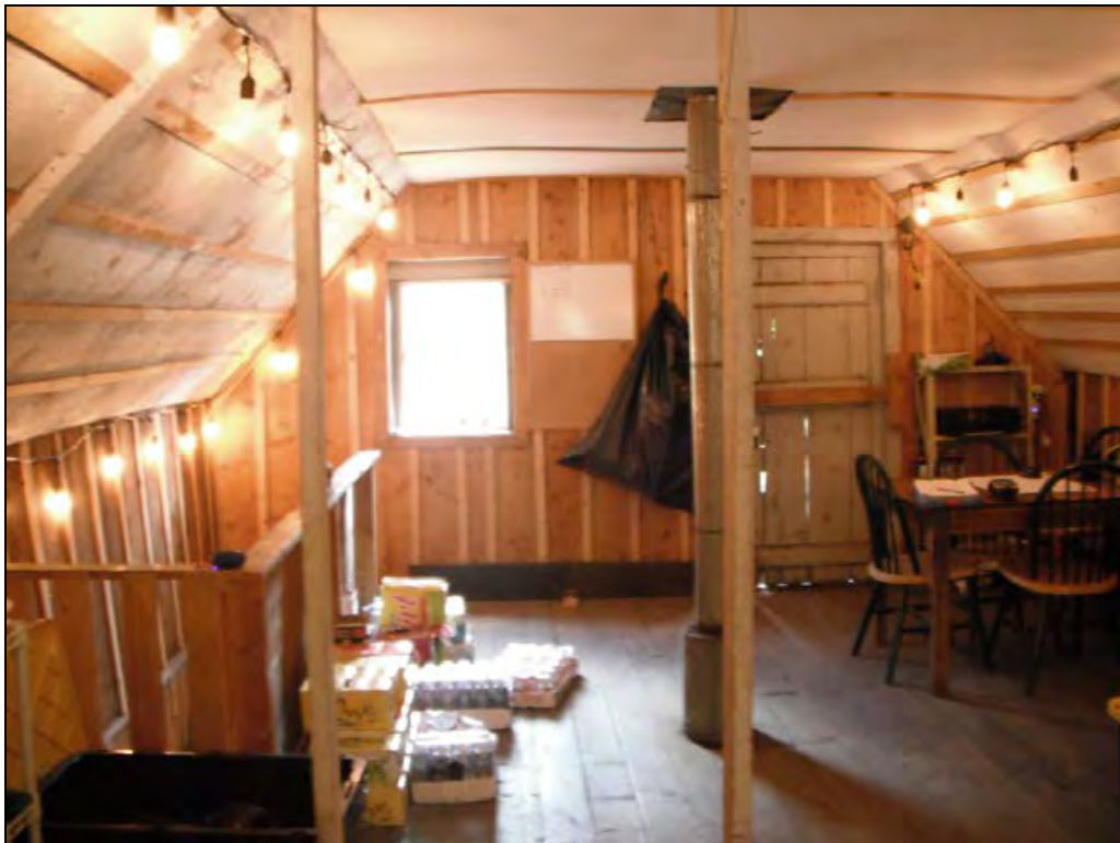
5GN6528 – General Store. View of the interior, south wall on the second floor. View south. (Roll 19-261, image 235, 09/27/2019)
