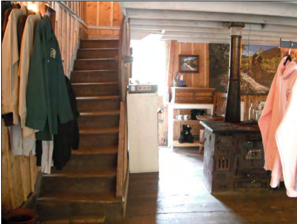
5GN6528 – General Store. View of the interior, stairs along the east wall and south wall. Note use wear on the stairs. View south. (Roll 19-261, image 232, 09/27/2019)
