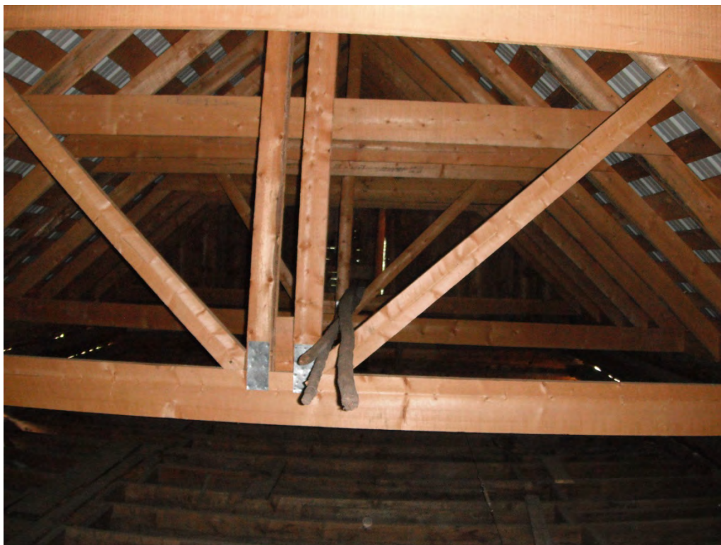
5GN6527 – Crystal Club. Interior, view of the new roof trusses above the main room of the original building. View north. (Roll 19-262, image 285, 09/27/2019)
