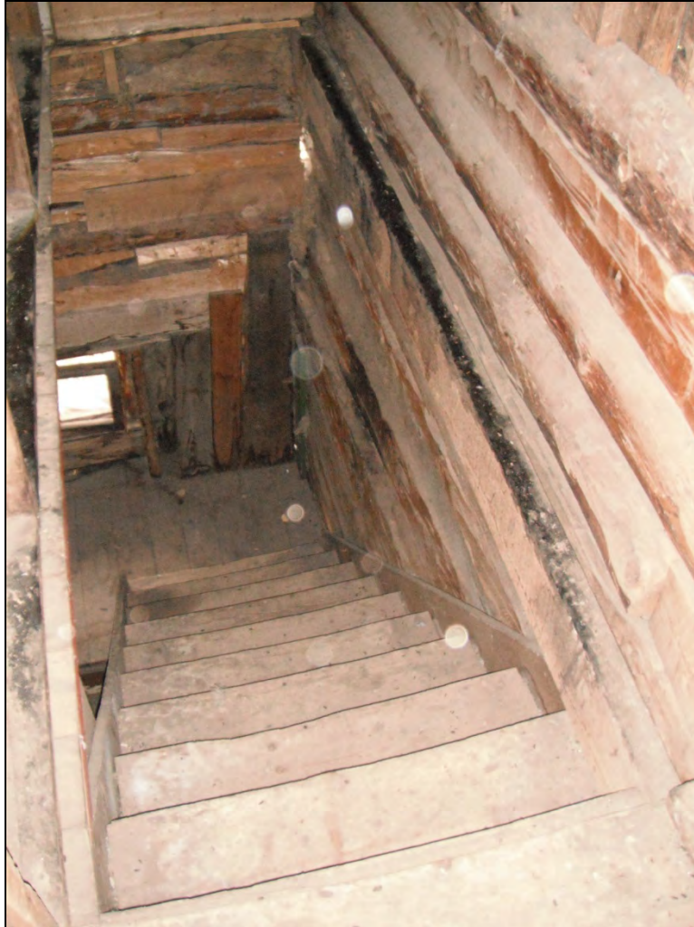
5GN6527 – Crystal Club. Interior, view down the stairs in the addition from the second floor. Note use wear on the stairs. View west/down. (Roll 19-262, image 295, 09/27/2019)
